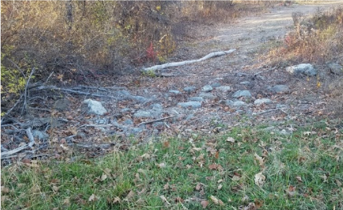
2020 WP-7 (east wall) crushed, was 1.5 feet tall
