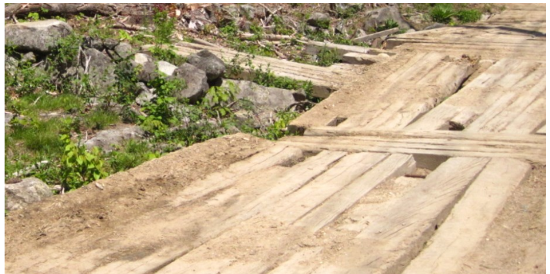
2020 support of timber mat was inadequate above WP-15
