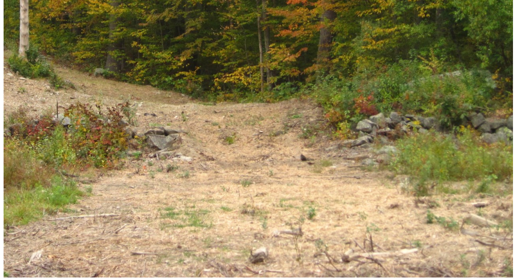
2020 breach is wider, wall damaged, stones missing
