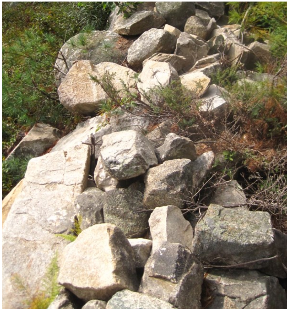
2020 north breach, now a pile of loose stones
