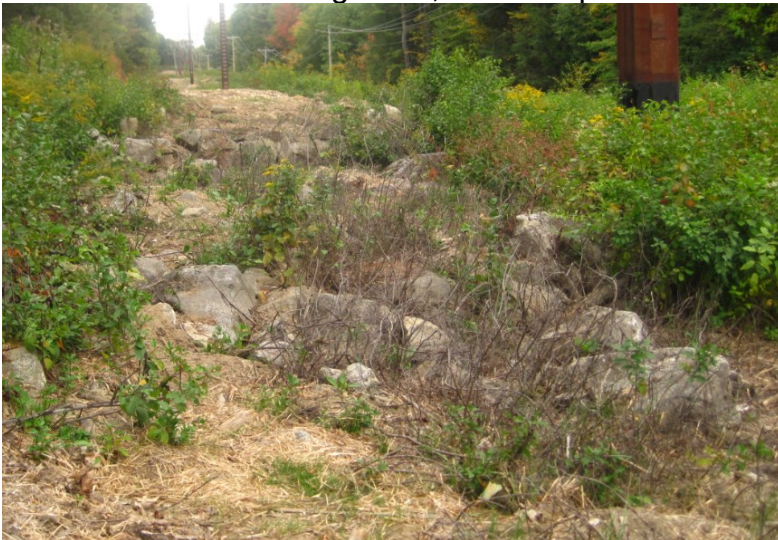
2020 WP-15 in the foreground, wall collapsed
