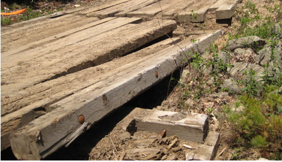
2020 timber mat support failure over the stone wall
